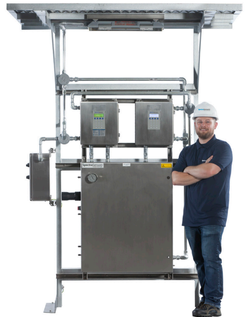
A gas analyzer shelter with a 2-Pack TDLAS analyzer mounted on a rack with a sunshade and fitted with fluorescent light and power distribution box
