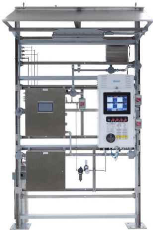
Gas analysis shelter with a Raman Optograf analyzer mounted on a rack with sunshade and fitted with a PLC, LED light, power distribution box, and fiber optic cable junction box.
